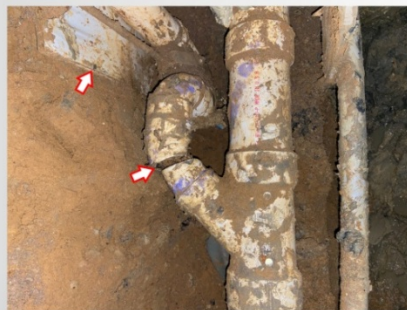
Plastic Panel Non-Isolated Void System and Cracked Plumbing
