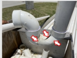
Multiple Cracks in P Traps
