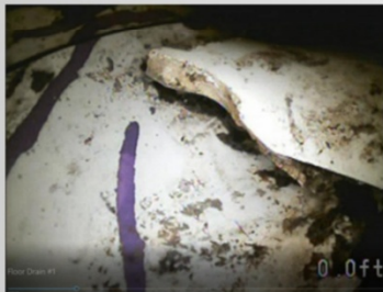
Close-Up View of a Cracked P-Trap Under a Floor Drain (No Trap Seal Due to Cracks)
